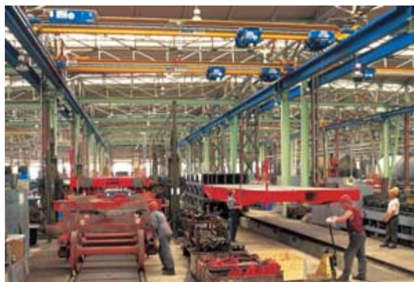
Two type E monorail hoists on type ELV single-girder overhead travelling cranes
